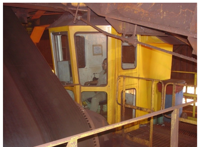
Fig. 3. Operation cabin of the tripper, with a local operator controlling the machine position in manual mode.
