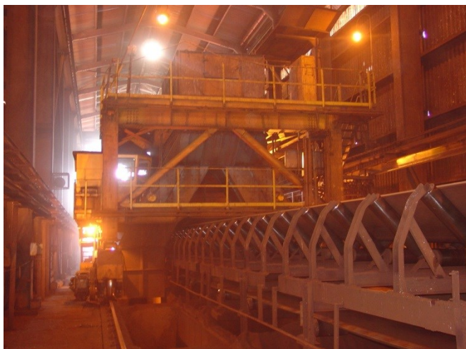
Fig. 2. Tripper of the Secondary Screening facility of the Carajás Iron Ore Processing Plant.
